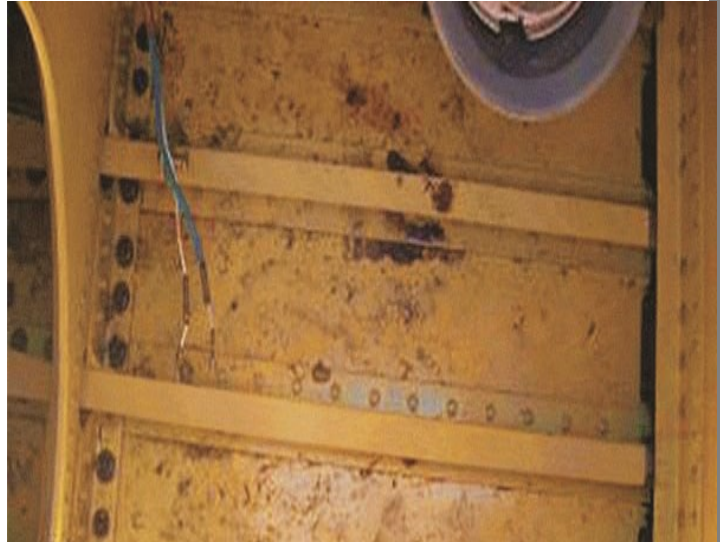
The brown-black debris on the bottom of this tank is made up of fungus and bacteria. This growth can clog fuel filters causing the airplane fuel quantity indication system to read incorrect values, and eventually cause structural corrosion of the aluminum stringers and wing skin. Credit: Boeing
